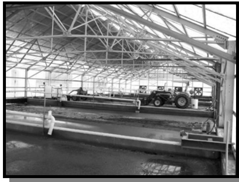
Town of Hanover Sludge Drying beds. Polymer feed tanks visible on left.
