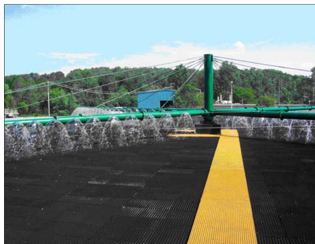
Completed Trickling Filter in Operation
